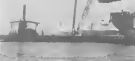
STEAM ENGINE putting No. 6 derrick barge hoists the second of four 60-ton desalters from the deck of the George Lyles. Problem was to keep the vessel from listing into the gantry.
